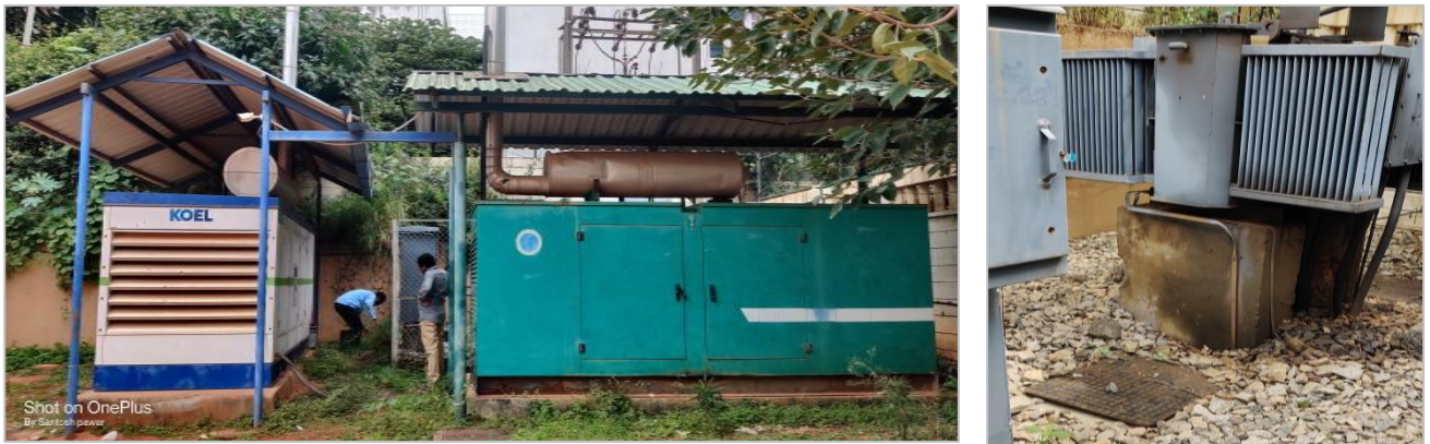
Investigative parameters – Ecological Management – Diesel Generator, earth pit areas for backup measures
